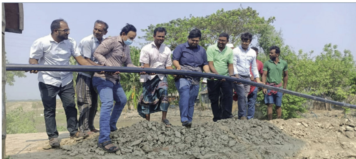
Figure 5: Chairman of Dumuria upazila, Khulna district, inaugurating the rehabilitation of a solar-powered piped water scheme led by the SafePani team in April 2022.
